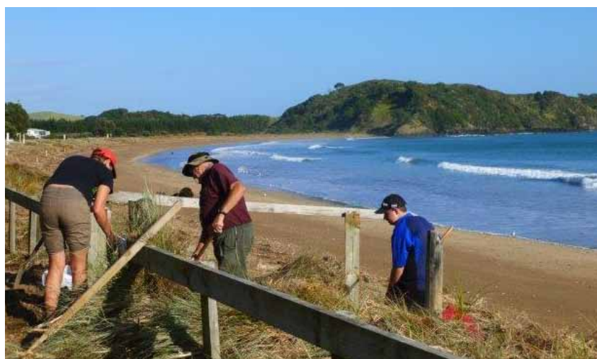
A working bee gets underway at Taipā to repair damage in the wake of two ex-tropical cyclones
